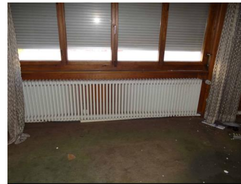
paint on radiator
